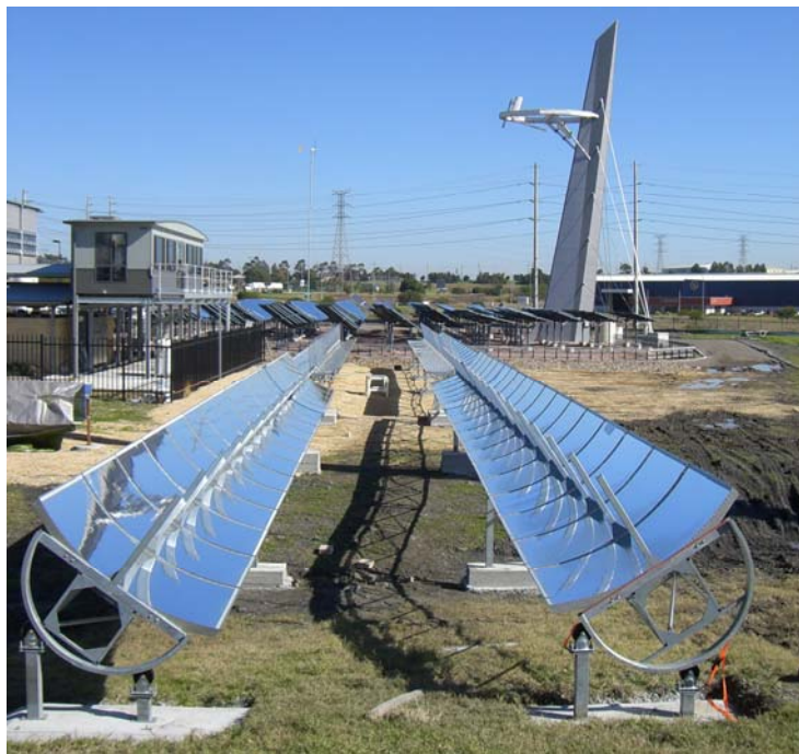
Figure 2.1 View of parabolic trough arrays at CSIRO
